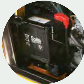
Rotational Battery Installation
